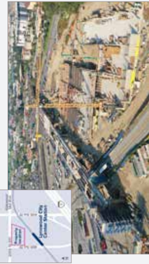
Drone image of the Lynnwood City Center Station construction, courtesy of Skanska Construction.
