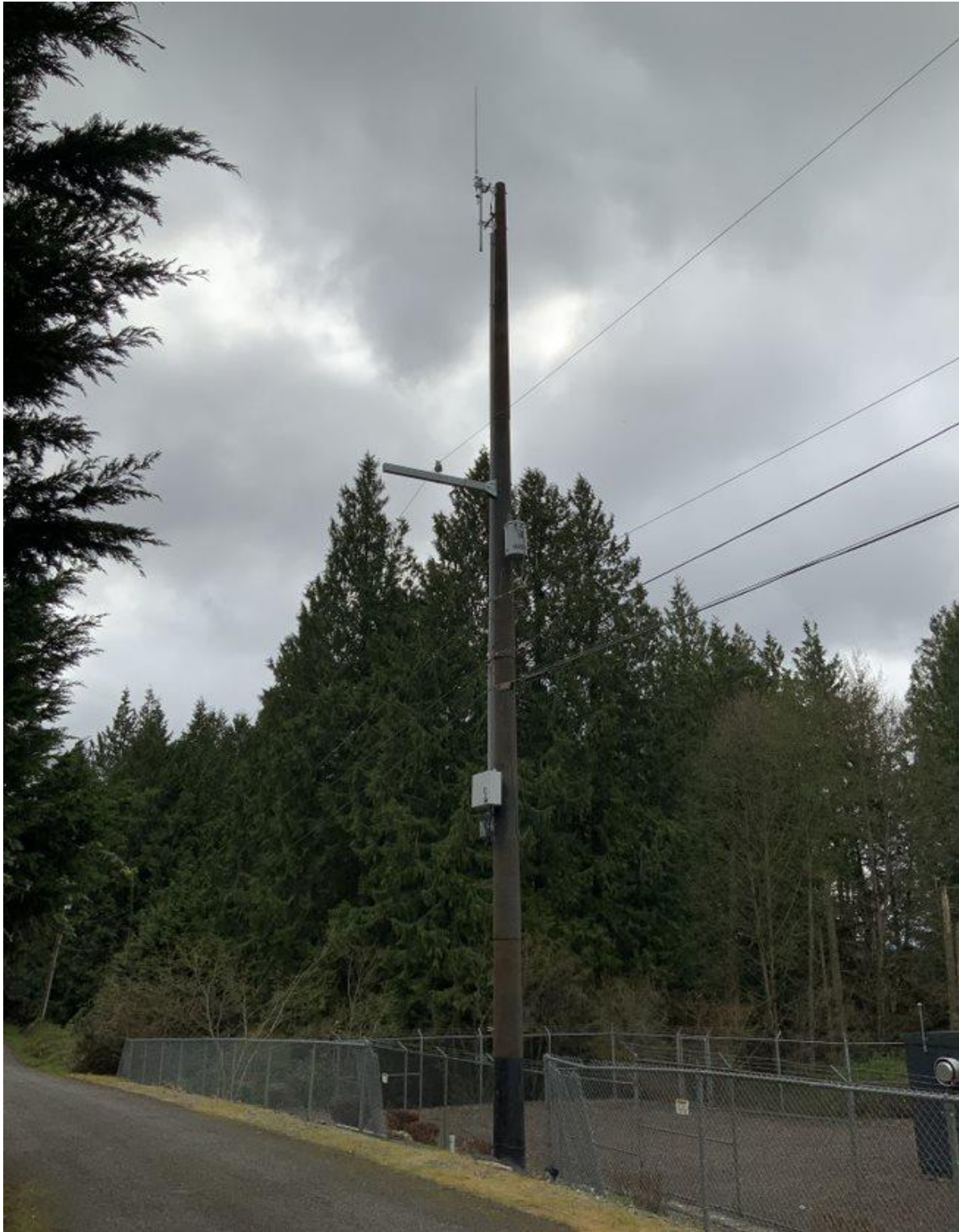
Figure 3. Example of AMI pole/base station/antenna installed at the Bunk Foss Substation site in Snohomish County.
