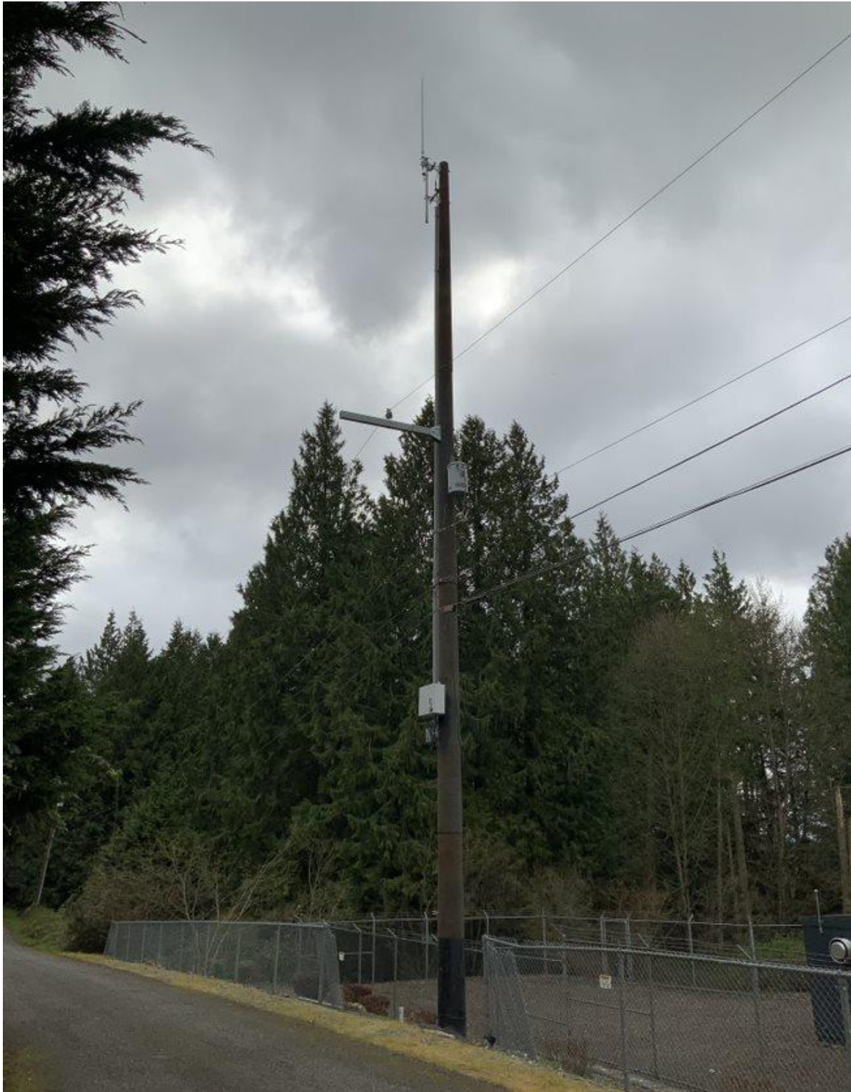
Figure 3. Example of AMI pole/base station/antenna installed at the Bunk Foss Substation site in Snohomish County.
