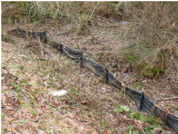
Photo 4-3. Septic system bypass.
