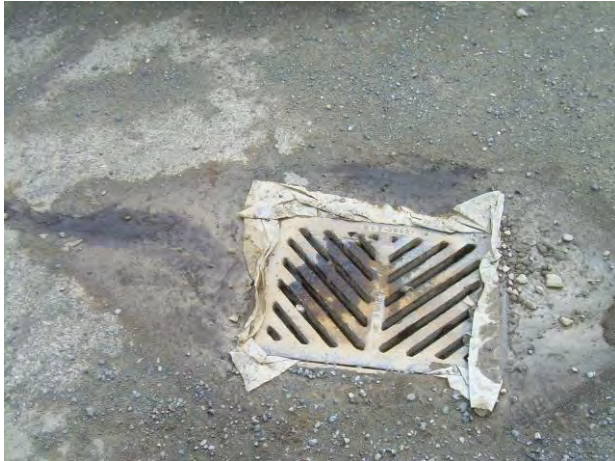
Photo 4-24. Oil spilled on catch basin blocked with plastic.
