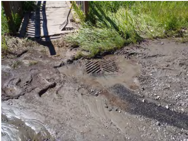
Photo 4-26. Water line burst and subsequent soil erosion.
