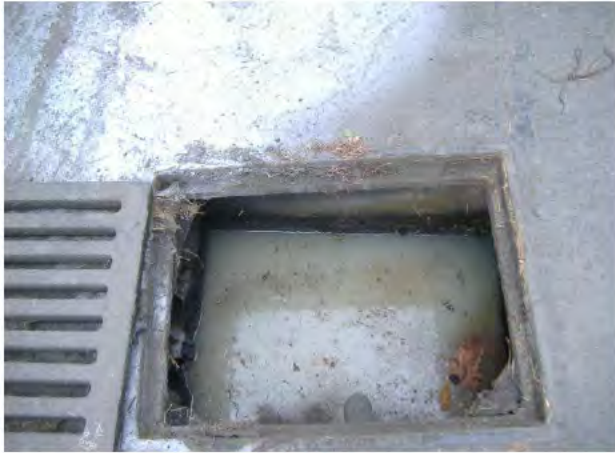
Photo 4-18. Grease in catch basin.
