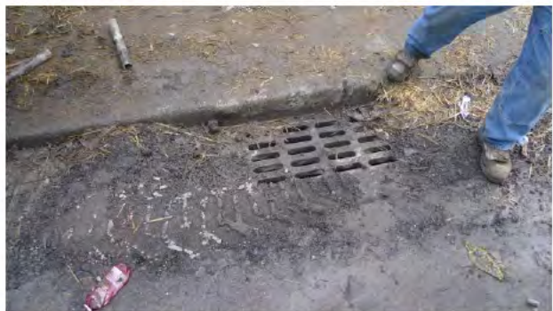
Photo 4-23. Catch basin without filter sock.
