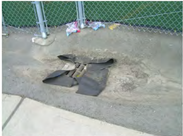
Photo 4-21. Functioning catch basin filter sock.
