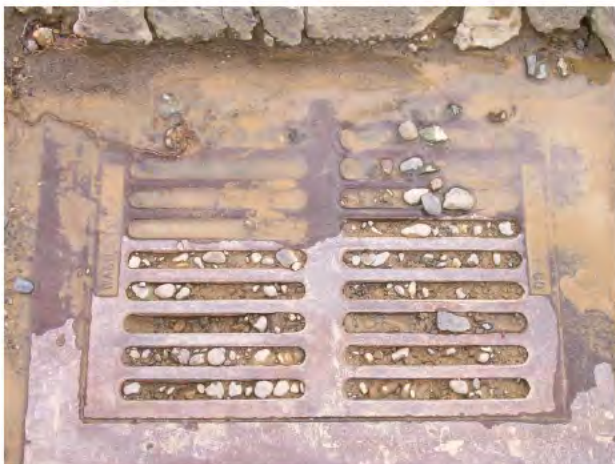
Photo 4-22. Catch basin plugged with sediment.
