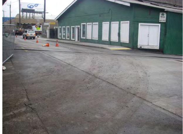
Photo 4-29. Construction entrance sediment trackout.
