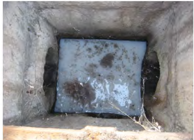
Photo 4-7. Paint in catch basin.
