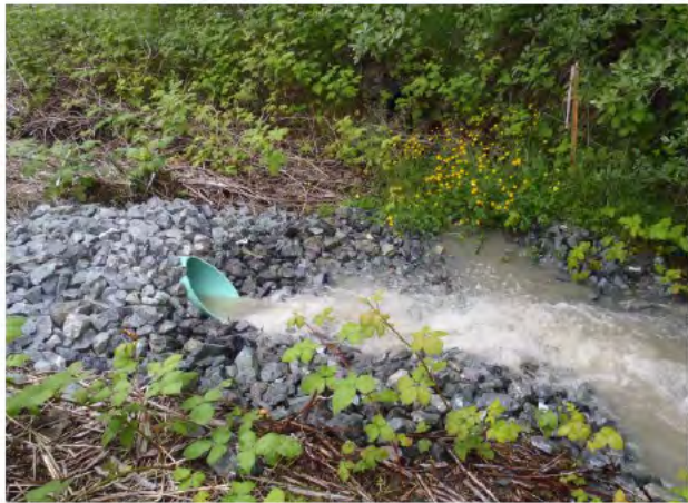
Photo 4-6. Downstream of sewer pipe blockage, flowing into wetland.
