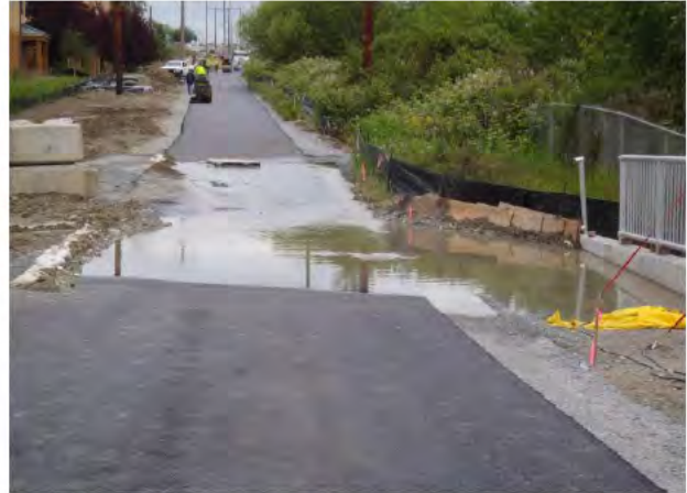
Photo 4-5. Sewer pipe blockage overflowing into catch basin.
