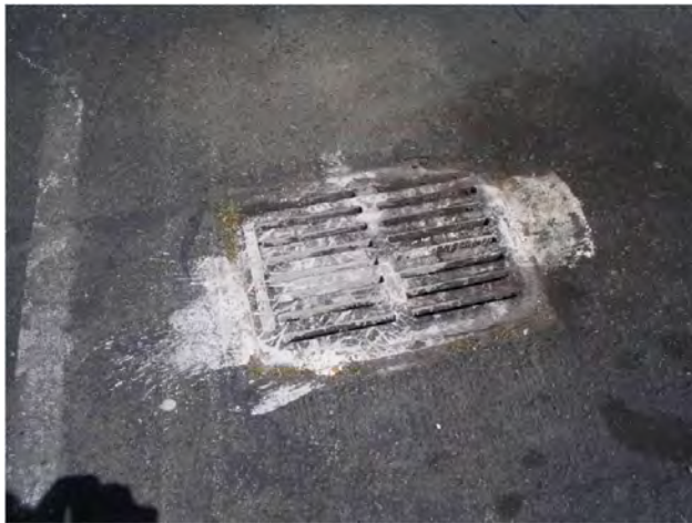
Photo 4-1. Paint dumped in storm drain.
