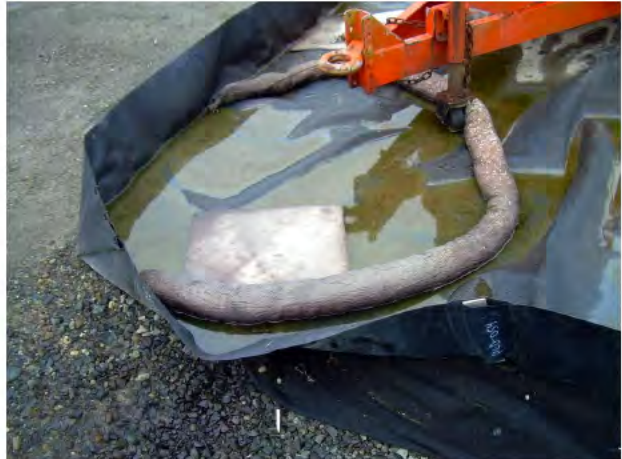
Photo 4-19. Leaking water pump in secondary containment.
