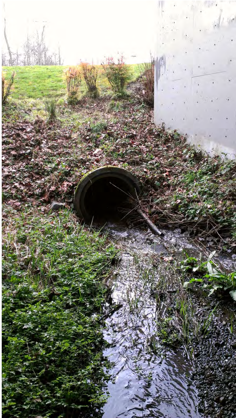
Photo 111: Golde Creek facing south, at 196th Street SW. Three foot concrete culvert crosses under 196th Street.
