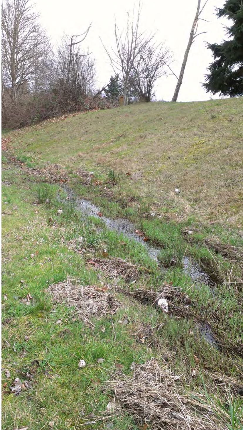
Photo 607: Ditch along the south side of Alderwood Mall Parkway, facing east. Ditch may flood during high intensity rain events in this location.
