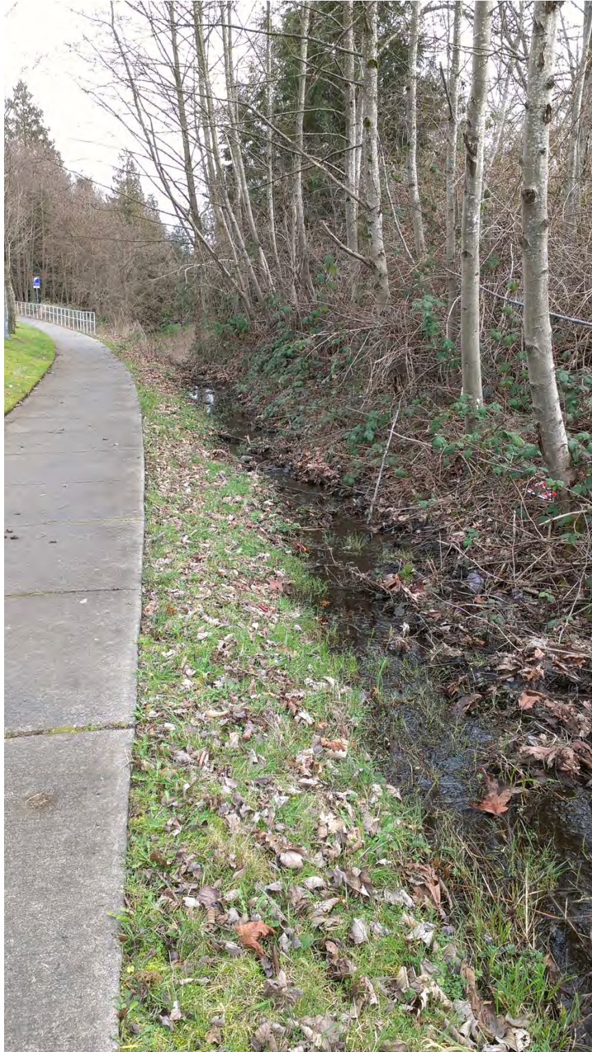
Photo 608: Ditch along the south side of Alderwood Mall Parkway, facing east. Ditch slope steepens in this area.
