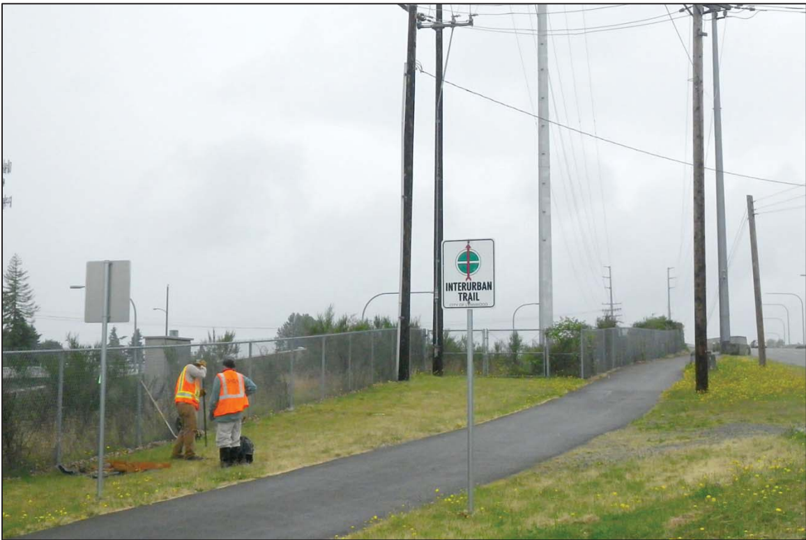
Figure 9. Overview of SP-8 along the Alderwood Segment of the Seattle-Everett Interurban Trail, view to the south-southeast.
