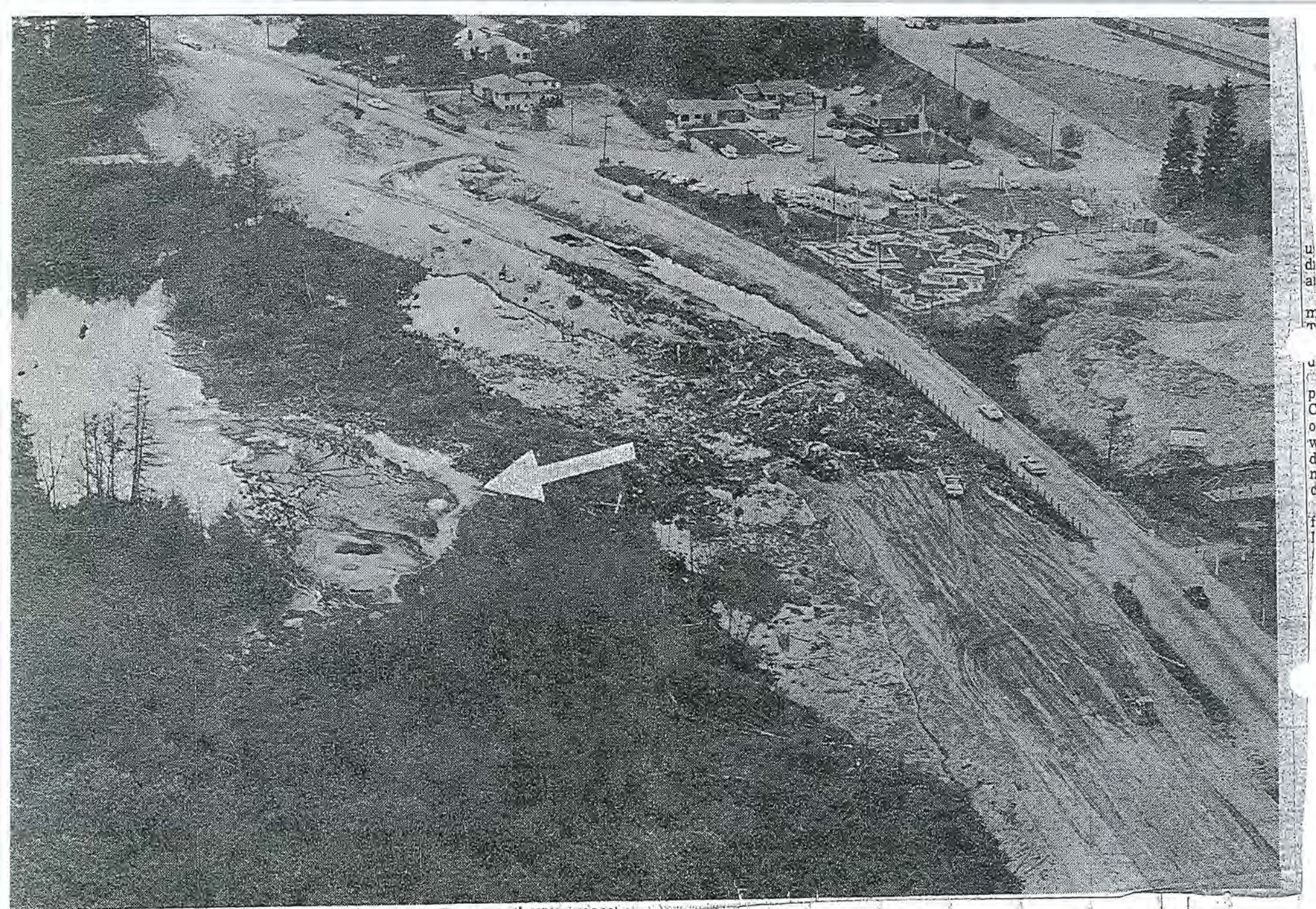
HAT SINKING FEELING —This is an aerial view of the project along 196th Street near Scriber Lake. Hundreds of truck-loads of broken wood have been used to fill the large hole in the road bed which appeared last spring. The arrow indicates the lake level. The bed sunk as much as 40 feet below the level of the lake. The weight of logs and sand in the road bed pushed much of soft bog below to the side. (Staff Photo by Pete Kinch, Courtesy of Cal-Aero.)
