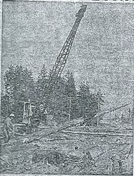
SWINGING into place is another huge log for Lynnwood area's new "skid road" base to highway improvement. It was preceded by an estimated 3500 Christmas trees.
