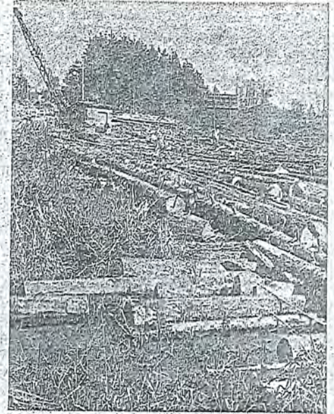
LOGS, logs everywhere look like the famed "skid road" of Seattle pioneer days. But Lynnwood road will have conventional paving-poured when this bog cover settles.
