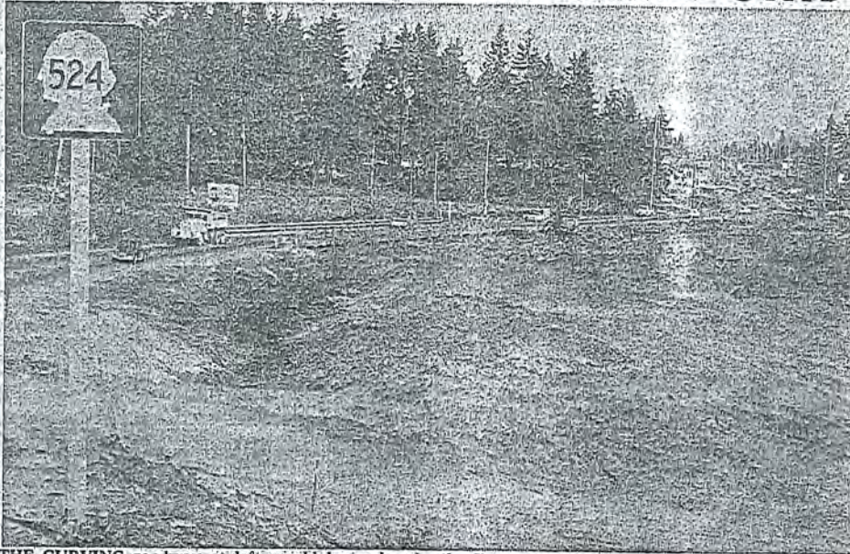
THE CURVING roadway at left would be replaced by a straight path from Lynnwood to Alderwood Manor when construction is completed, possibly this summer. Also underway is connecting roadway to
