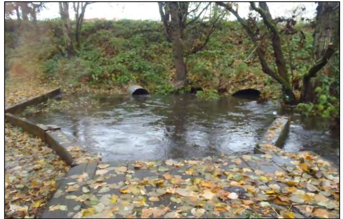
November 23, 2011 flooding at the diversion weir.
