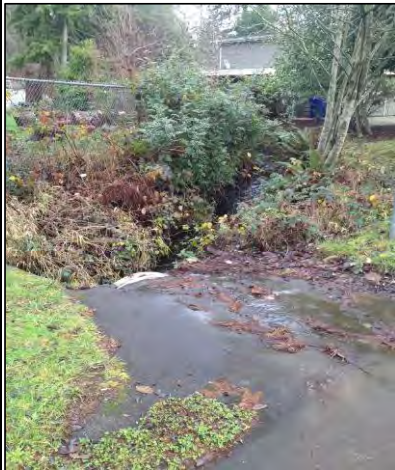
Looking upstream to existing channel and culvert inlet at 191st ST SW.
