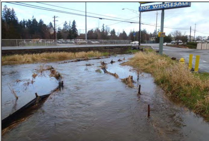
March 14, 2011 Flooding near Flynn's Carpets.
