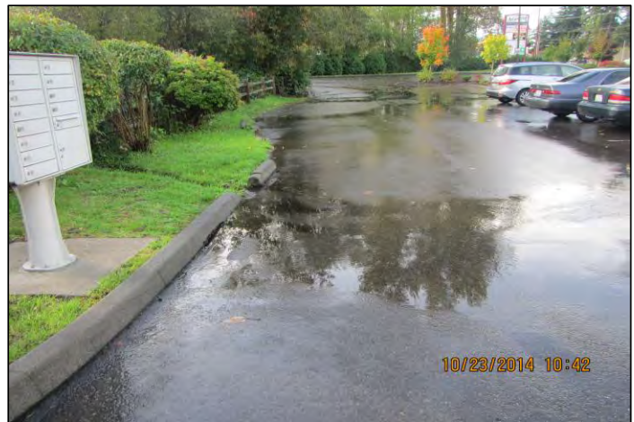
Parking lot near Eunua Plaza overlying one of the existing driveway culverts.
